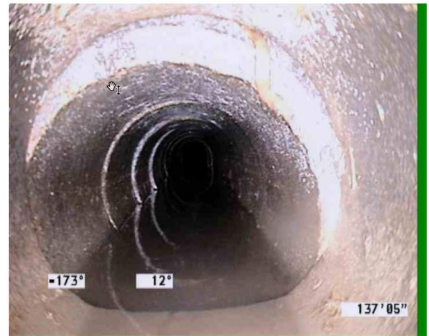
1, 00:05:35, 137.70ft Joint Offset Large, 1Inch
